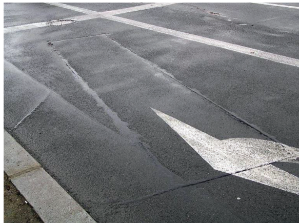
Fig. 2 Induction loop in a left turning lane [4]
