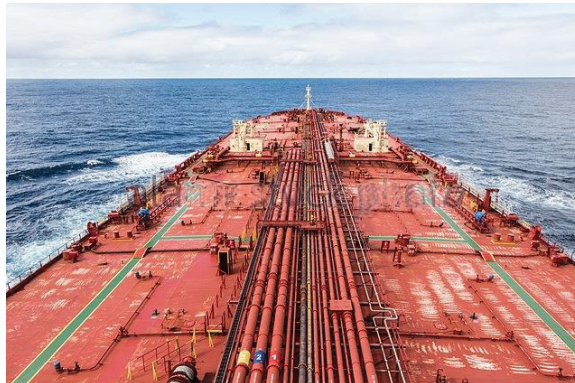
Fig. 5 Pipelines on a tanker [11]
